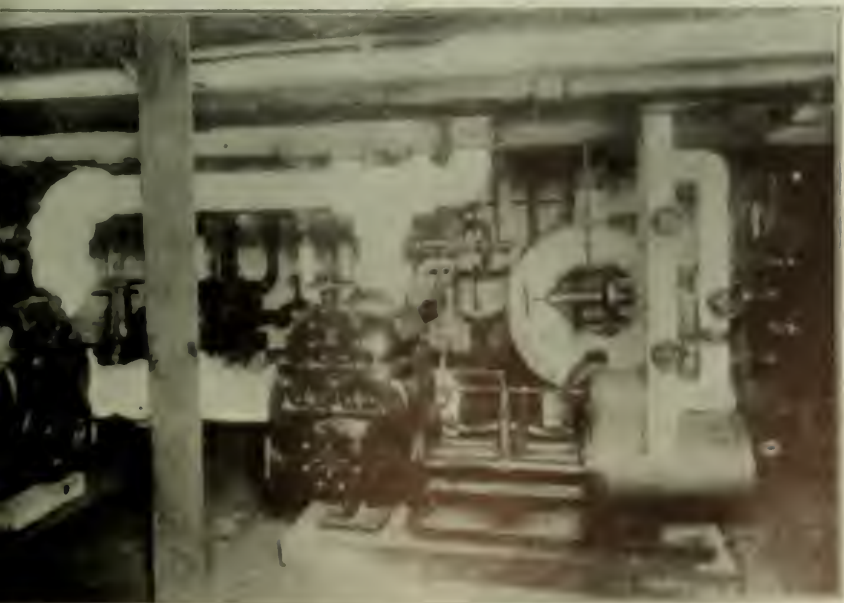
FIG. 10. A PORTION OF THE STEAM PUMP
